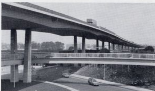
Hi-Build Chlorinated Rubber Paints and Pitaguard Pure Phenolic Micaceous Iron Oxide Coatings were used to protect the main structure and parapets at the Staples Corner fly-over. (Photograph by courtesy of PFA, Central Electricity Generating Board and Department of Transport).
