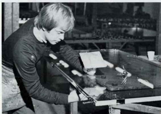
Evode's Epoxy Polysulphide Sealant 2793 being applied to a double glazing unit at Anglian Windows Limited.
