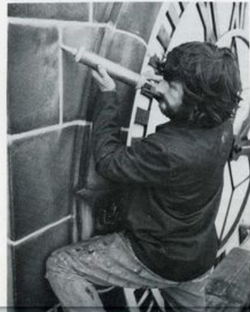
Evode Potevo two-part polysulphide sealant being gun-applied to joints between slabs of Lancashire Grit Stone on the Lancaster Town Hall Clock Tower, by the Evode Joint Sealing contract team.
