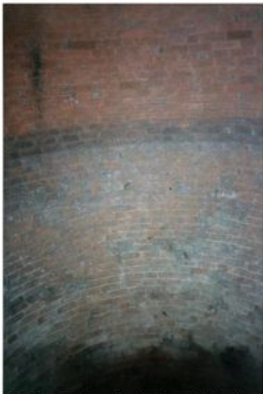
The brickwork of The Ice Chamber seen from the doorway. Note the change in colour of the brickwork caused over the years by contact with the ice stored there. Photo John Walker 1992.
