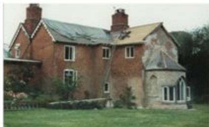
The Garden House. A new wooden barge board was put up, with the same striking pattern as the old disintegrating barge board.
