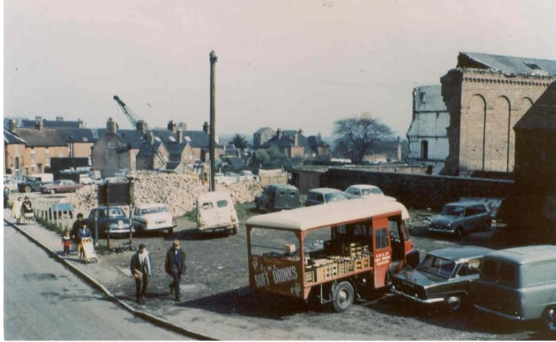
Buntings old Brewery building being demolished seen from the first floor window of The Beehive, Bradley Street.
